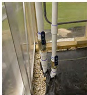
Dual water lines
