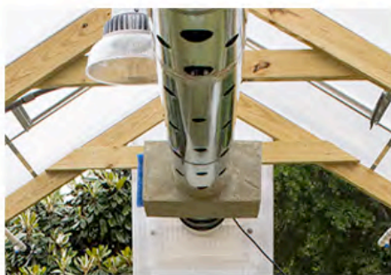
LED fixture, and airflow ductwork
