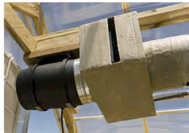
Exhaust fan and filter box
